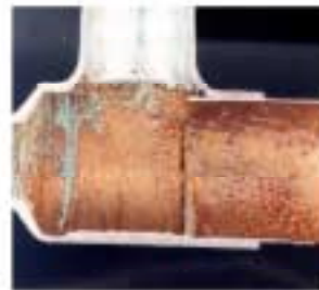
Erosion-corrosion of copper water pipe
