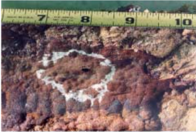
External corrosion on ductile iron pipe
