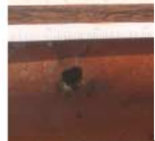
Stray current corrosion
